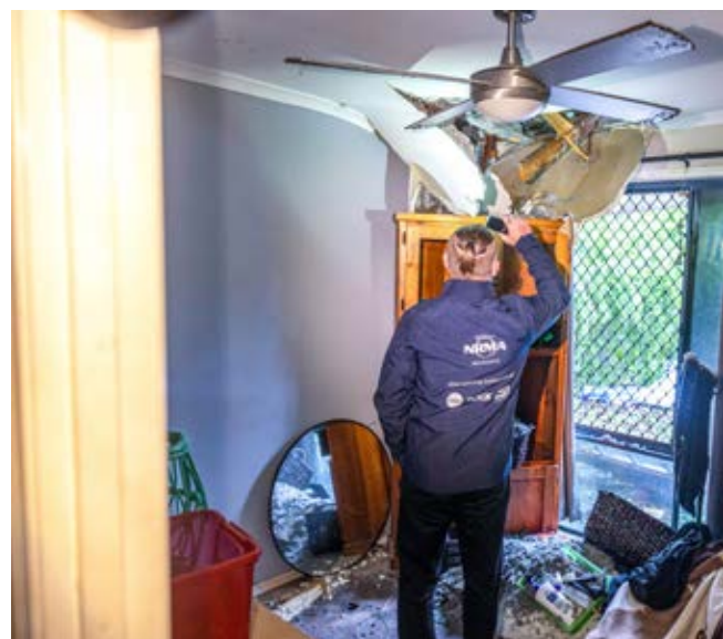
TOP & MIDDLE: Tropical Cyclone Narelle home damage; BOTTOM: NRMA Insurance assessor visiting damaged home in Queensland, Tropical Cyclone Alfred.
