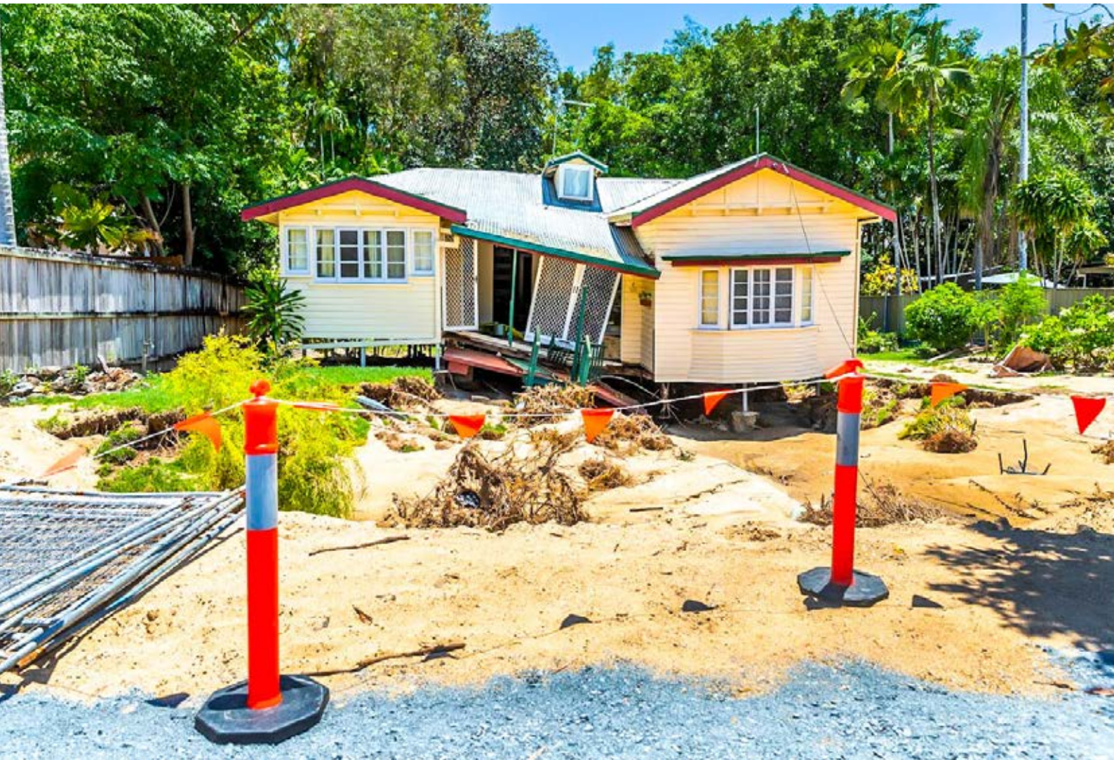
Far North Queensland home impacted by Tropical Cyclone Jasper
