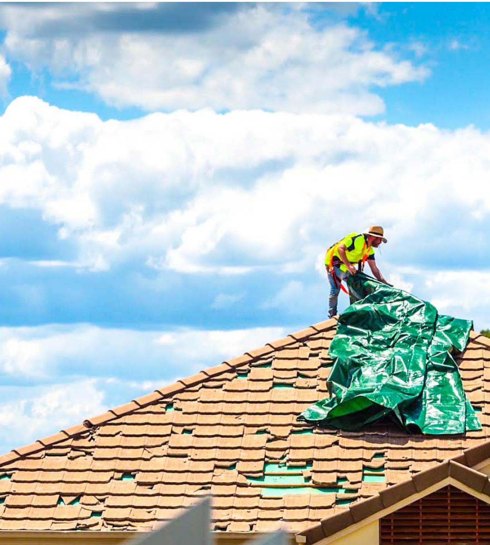
South East Queensland home impacted by a hail storm, 2020
